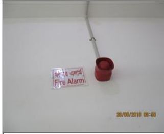
Photo of fire safety equipment Fire alarm.JPG
