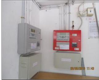
Photo of fire safety equipment Control panel.JPG
