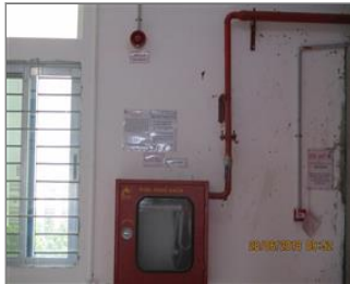
Photo of fire safety equipment Fire hose cabinet.JPG
