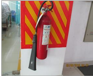
Photo of fire safety equipment Fire extinguisher.JPG
